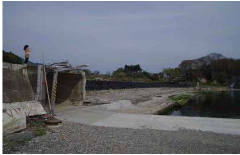
Destroyed seawalls by the tsunami
